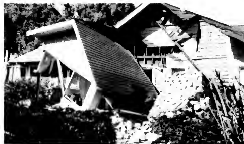
Photo 3. One of the many chimneys that collapsed. In this house, support for porch also fell. Photo courtesy of City of Los Angeles Department of Building and Safety.
